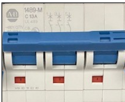
Bank 1 Breaker Closed/Hot
