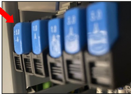
Bank 3 Breaker Tripped
