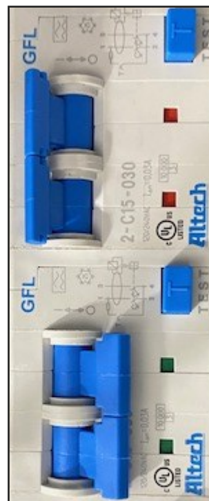
Bank 3 Breaker Closed/Hot (ON)
