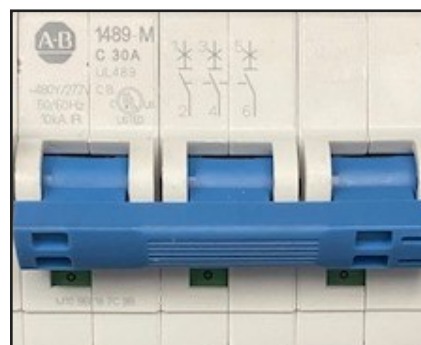
Bank 1 Breaker Open/Tripped
